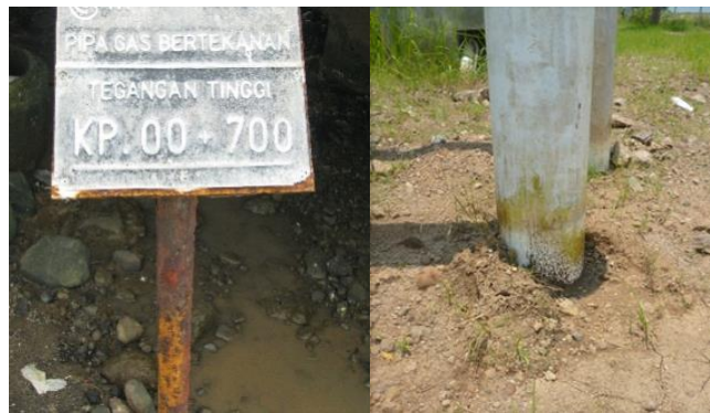
Figure 1: (a) Buried pipeline and before road crossing ; (b) Pipeline arise after buried
